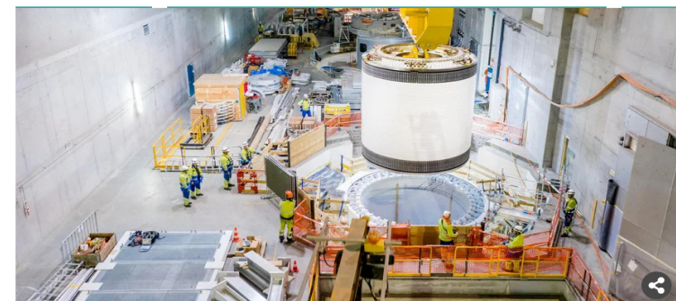
▲ Building the engine room at Nant de Drance power plant Nant de Drance / Sébastien Moret
